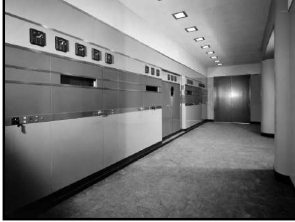
RCA even carried its streamline moderne styling to its line of transmitters, as is evident in this RCA high-power shortwave transmitter circa 1940.
